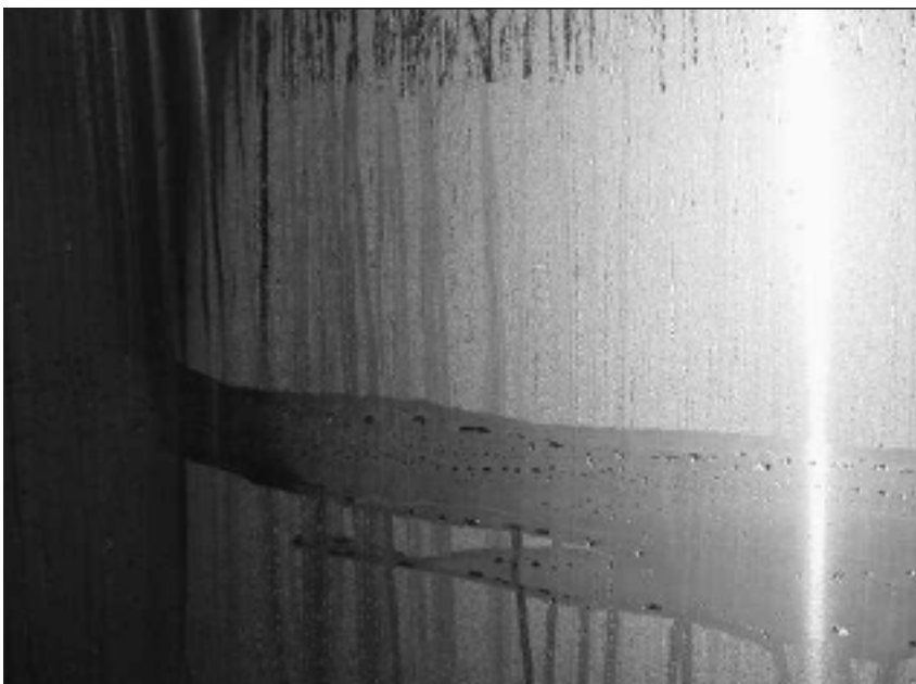
Figure 6 – Heavy Water Condensation on a Coil
